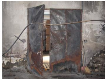
Non fire rated door – exposed side
