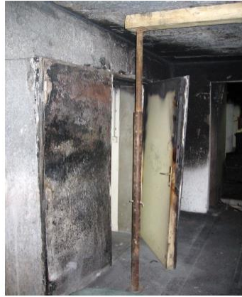
Fire rated door – exposed side
