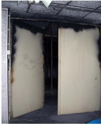
Fire rated door – non exposed side
