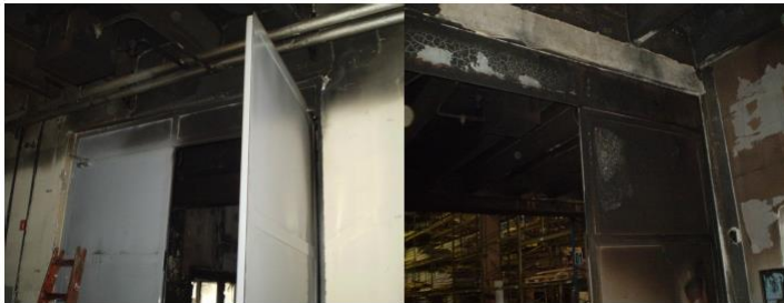
Fire rated door – non exposed side
