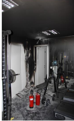
Fire rated door – exposed side
