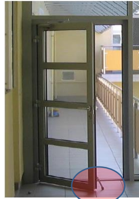
Fire rated door
