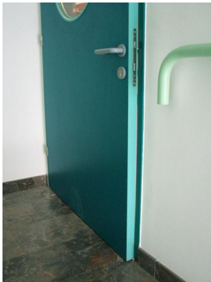
Fire rated door
