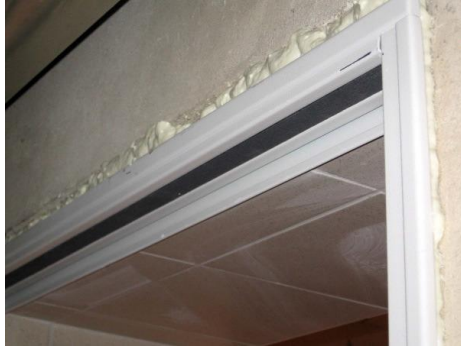
combustible gap filler on a fire rated glass
