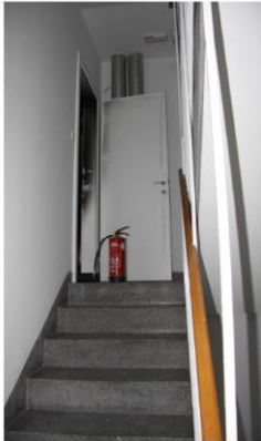
Fire rated door – non exposed side
